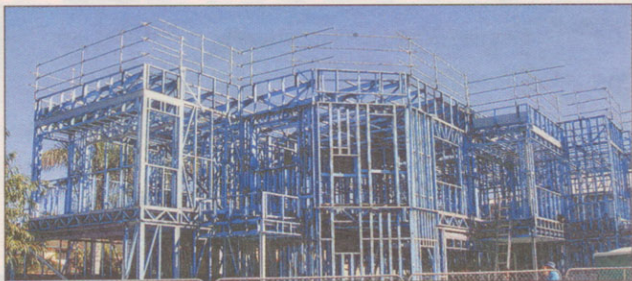
A 21st Century Steel Homes' frame takes shape on this Gold Coast project
